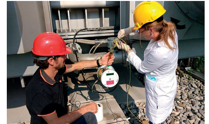
On-site validation of moisture and dissolved-gases-in-oil on-line monitoring sensor
